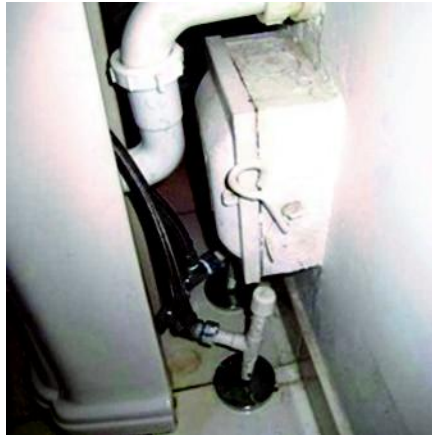
Who's going to work on this.....if there is an electrical or plumbing problem ???
