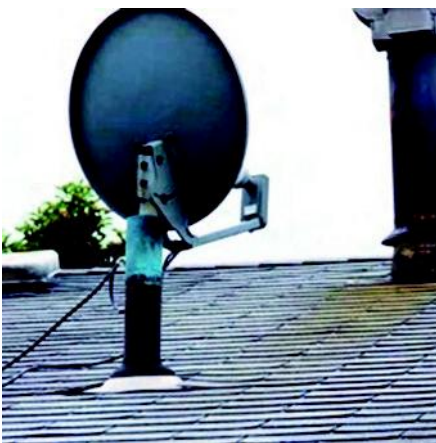
Can't mount it on the roof....so let's just stick it in the venting pipe
