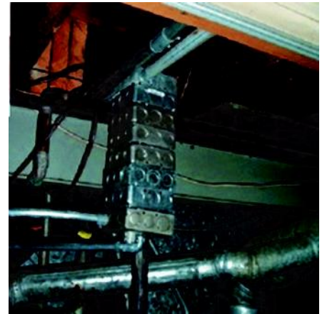
Missed it by a foot, why not use a bunch of spare electrical boxes?
