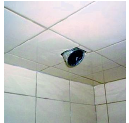
The ceiling was too low by a foot
